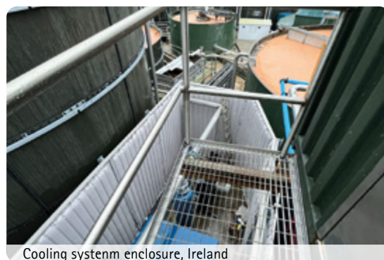
Cooling system enclosure, Ireland
