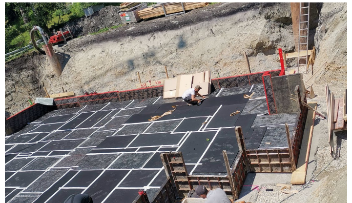
Semi-detached house in Gröbenzell, Cimax® is installed under the load-bearing walls due to groundwater
